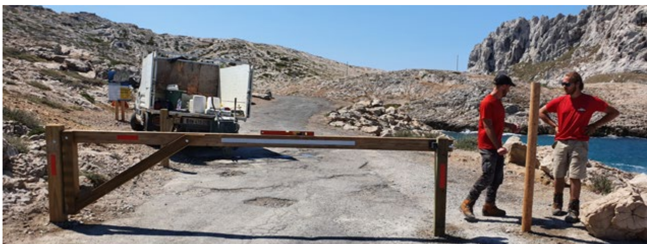
Unorganised parking on sensitive coastal habitats in Cap Croisette, summer 2020 (top), installation of a motor vehicle traffic restriction barrier (bottom), summer 2021
